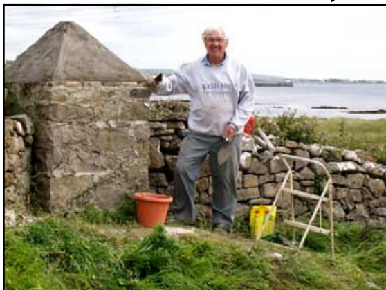
Never happier than when out working in the fresh air. Dad repairs the dry stone wall outside my house
